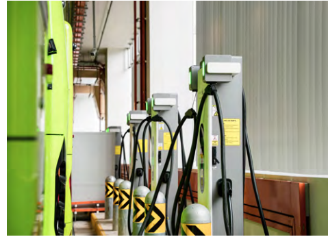
EV charging infrastructure at Gali Batu Bus Depot.
