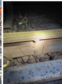
Rail breaks (25 nos.)
